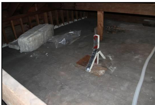
Beacon to identify access hatch to ballroom ceiling
